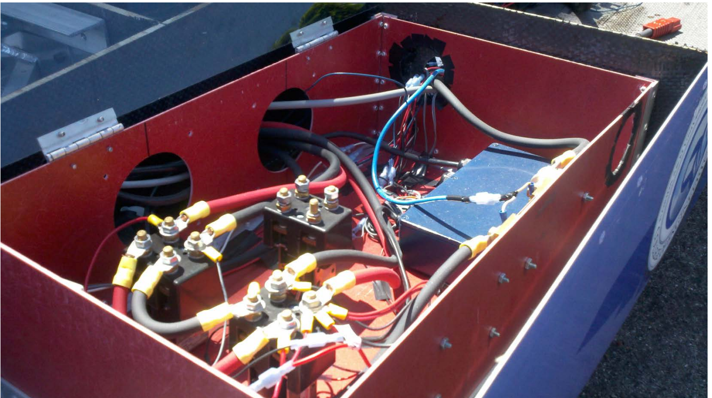
Figure 3.7.1 – The high power components are protected by a fiberglass box
